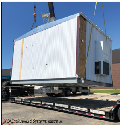
FIGURE 4. Prefabricated buildings, such as the control room shown here, may be prepared off-site and installed later
