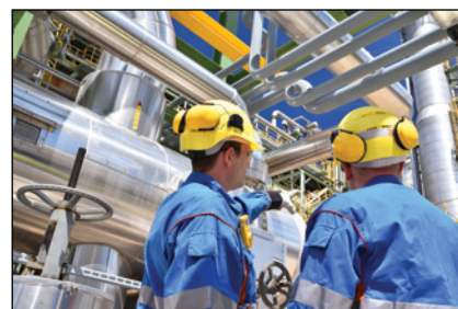
FIGURE 2. Improvements in equipment may require changes to the plant’s infrastructure
