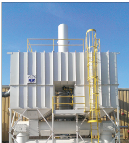
FIGURE 1. This two-canister regenerative thermal oxidizer (RTO) is equipped with high-cycle horizontal poppet valves
