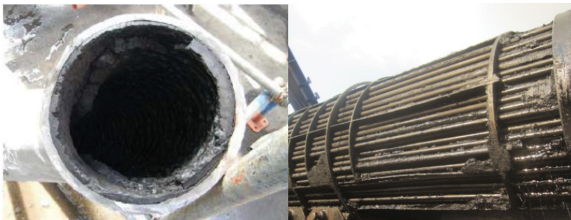
FIGURE 1. The photo on the left shows the inner pipe wall of a severely fouled fuel oil line. The photo on the right shows a tube bundle heavily fouled by asphalt and coke. Both examples are non-idealities illustrating why ideal hydraulic models deviate from reality
