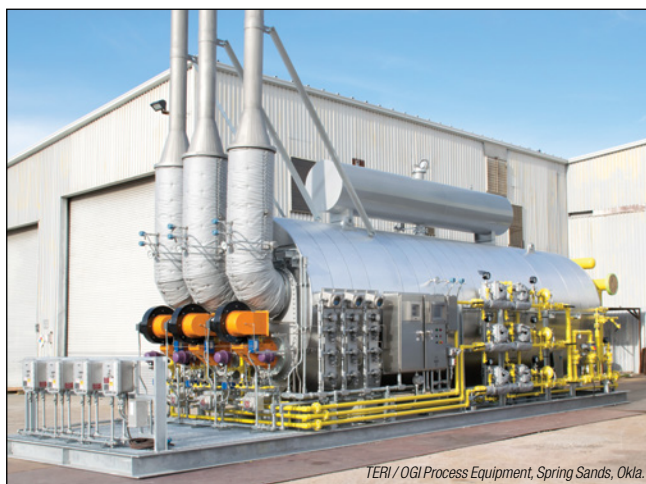
FIGURE 3. Process outages are required to install new equipment, such as the heater shown here
