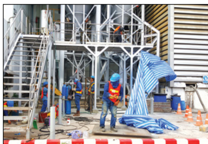
FIGURE 1. It is often the case that making improvements to CPI facilities is more cost-effective than replacing them
